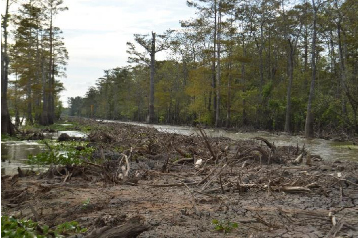
Fig. 3-E. This photo depicts illegal fill/Clean Water Act violations created by dredged material/dirt/spoil and debris remaining along the pipeline right-of-way after construction and pipeline markers placed inside new spoil created by BBP. Dirt seen in the adjoining the forest to the right side of the photo may likely have been the result digging/dredging during high water without any erosion control. Dean took this photo facing west/northwest at a location west of Cross Bayou, between the following approximate coordinates: 30°05'12.84" N, 91°22'38.47" W and 30° 05'10.71" N, 91° 23'51.29" W.
