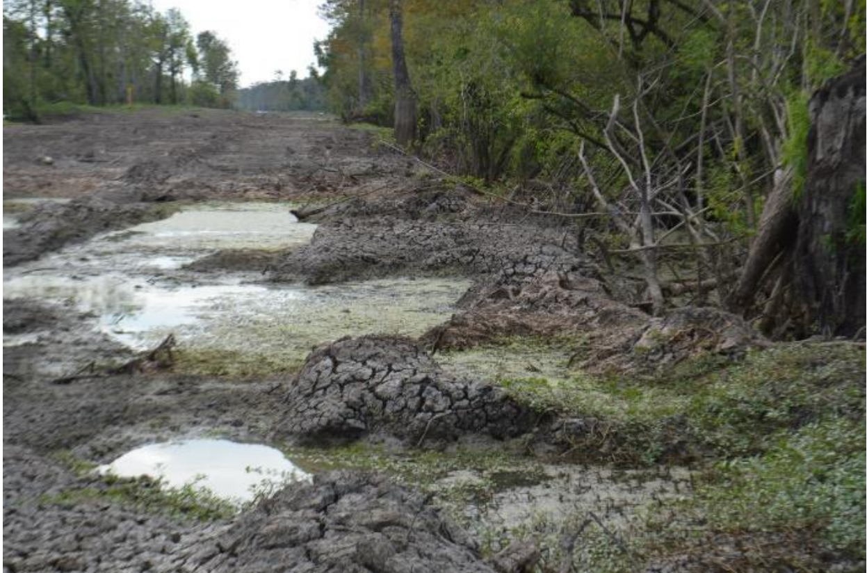
Fig. 1-E. This photo depicts piles of dredged material/dirt/spoil and large holes remaining after pipeline construction, in violation of the permit. Dean took this photo facing west from the banks of Cross Bayou, at the following approximate coordinates: 30°05'12.84" N, 91°22'38.47" W.
