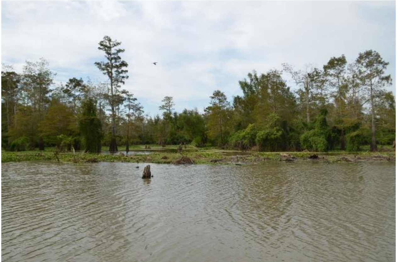
Fig. 5-E. This photo depicts a pre-existing, unnamed slough along the right-of-way that is dammed/blocked by construction-related debris, in violation of the permit. Dean took this facing north, at a location west of Cross Bayou between the following approximate coordinates: 30° 05'12.84" N, 91° 22'38.47" W and 30° 05'10.71" N, 91° 23'51.29" W.
