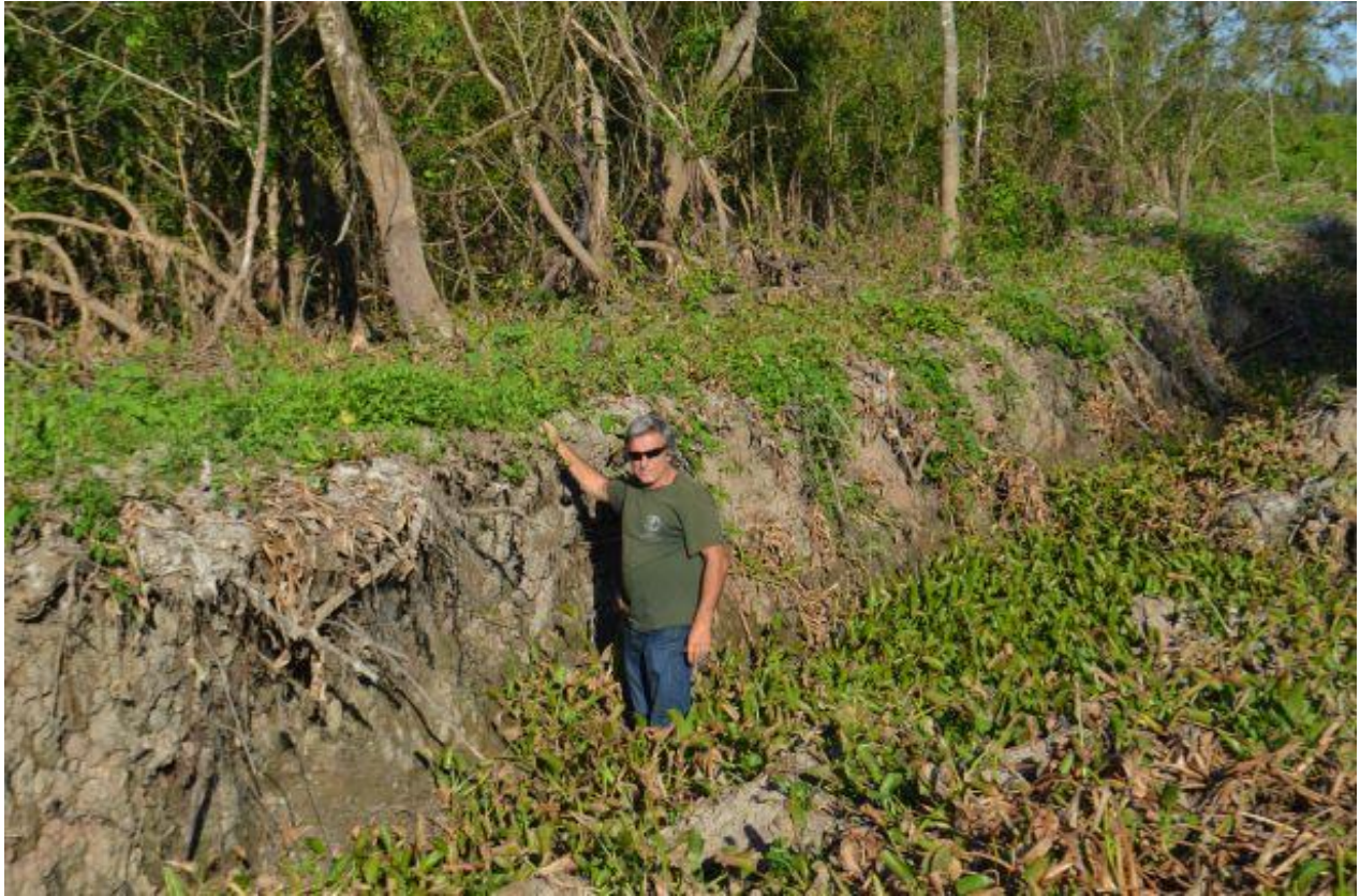
Fig. 7-W. This photo was taken by Shane Doucet during the September 11 monitoring trip. This photo depicts a large rut approximately 6' deep in the pipeline right-of-way, remaining after construction of the Bayou Bridge pipeline. Shane took this photo facing southwest very close to the dike that separates the canal to Bayou Chene, at the following approximate coordinates: 30° 07'20.8" N, 91° 33'49.4" W.
