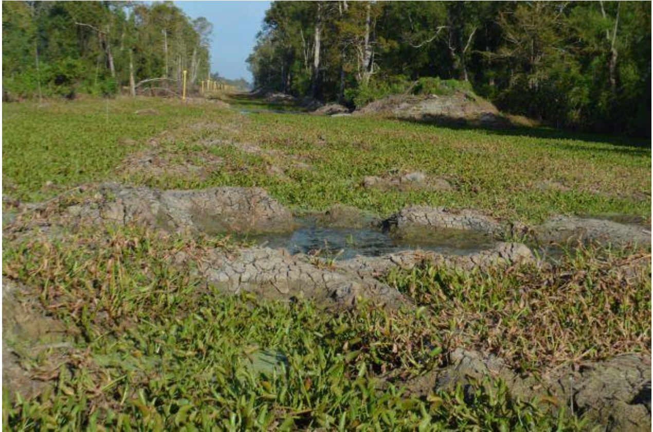
Fig. 4-W. September 11, 2019. This photo depicts piles of dredged material/dirt/spoil, including a large hill of dredged material to the right of the pipeline markers and channel, and large holes at the forefront remaining after pipeline construction, in violation of the permit. To the left of the photo, before the pipeline markers placed in elevated spoil, the pipeline trench is full of water and covered with water hyacinth, indicating that the pipeline appears to be uncovered or insufficiently covered at this location. This photo was taken from the west bank of Beau Bayou facing northwest, at the following approximate coordinates: 30°08'10.99" N, 91°35'48'68" W.
