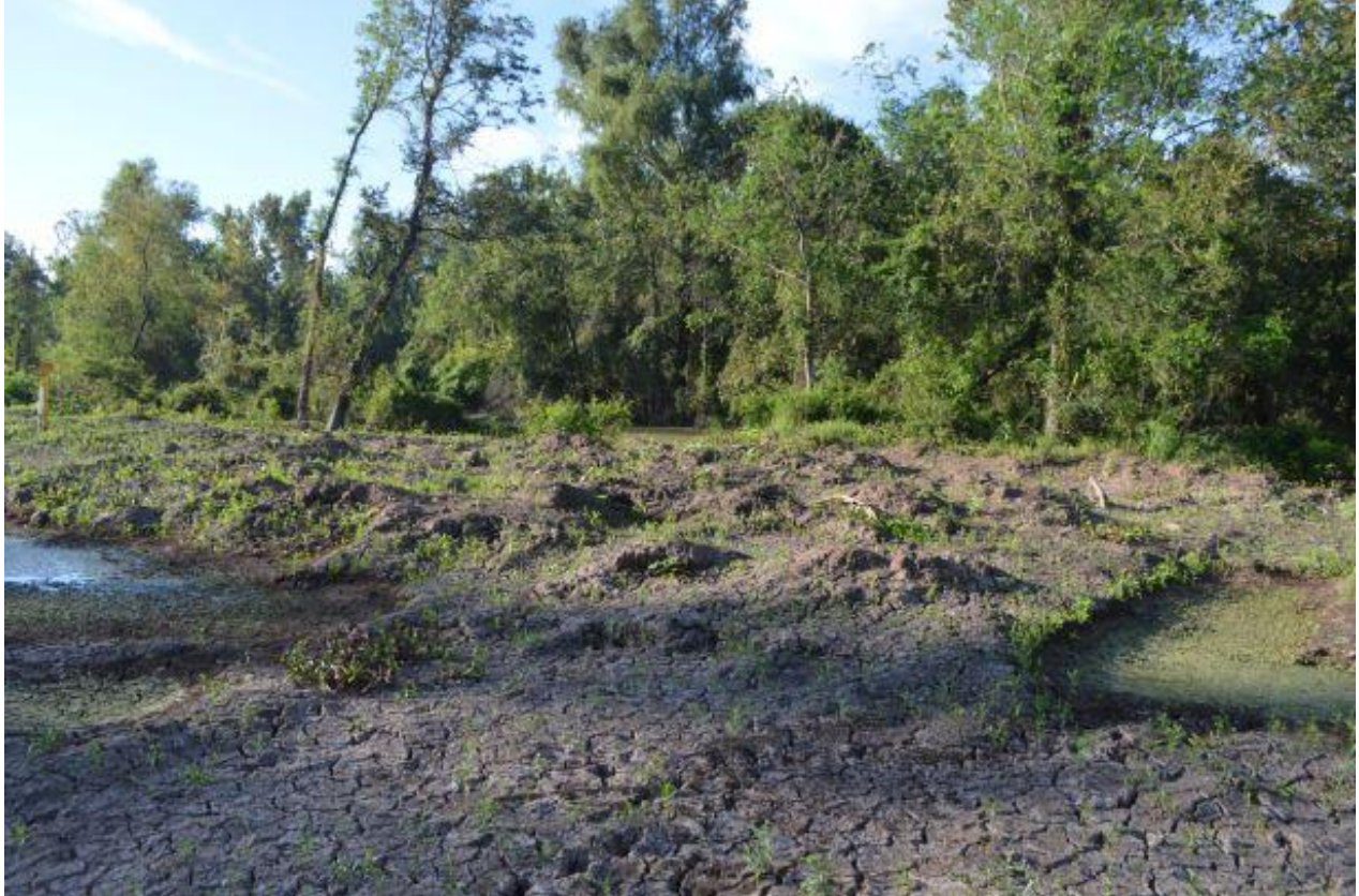
Fig. 6-W. September 11, 2019. This photo depicts yet more piles of dredged material/dirt/spoil and holes along the pipeline right-of-way, in violation of the permit. The pipeline trench is located in the lower portion of the photo, with water in the trench and what appears to be uncovered pipeline to the left side. Dean took this photo facing northwest between Beau Bayou and Bayou Chene, between the following approximate coordinates: 30° 08'09.66" N, 91° 35'46.74" W and 30° 07'20.8" N, 91° 33'49.4" W.
