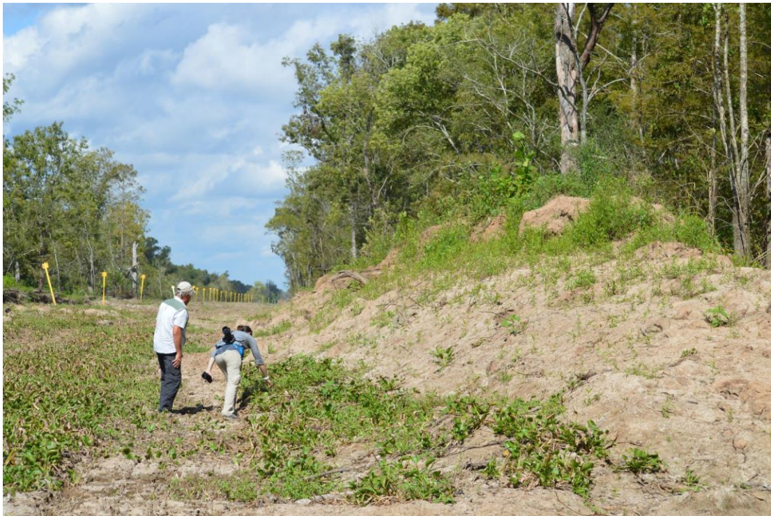
Fig. 2-W. September 27, 2019. This photo depicts illegal fill/Clean Water Act violation along the pipeline right-of-way. The pipeline is on the lower part of the picture without markings. The picture was taken facing northeast, approximate coordinates: 30° 07'38.37" N, 91° 34'27.79" W.
