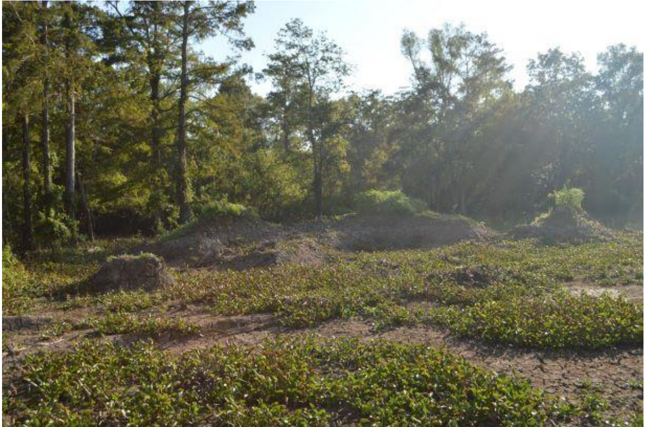
Fig. 5-W. September 11, 2019. This photo depicts more dredged material/dirt/spoil left along the pipeline right-of-way, in violation of the permit, with the pipeline located near the bottom of the photo without pipeline markers. Dean took this photo facing northeast between Beau Bayou and Bayou Chene, between the following approximate coordinates: 30° 08'09.66" N, 91° 35'46.74" W and 30° 07'20.8" N, 91° 33'49.4" W.
