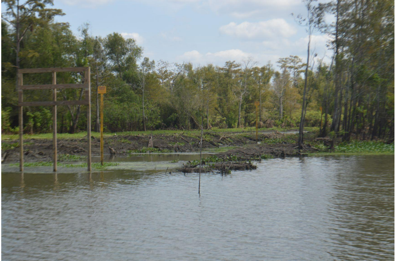
Fig. 9-E. This photo depicts markers in a the flooded pipeline trench, suggesting that in portions where the pipeline trench remains inundated with water at such a low water stage that the pipeline in these areas is uncovered or insufficiently covered per the terms of the permit (minimum of 4' cover). Dean took this photo facing northeast, at the following approximate coordinates: 30°05'16'61" N, 91°22'18.23" W.
