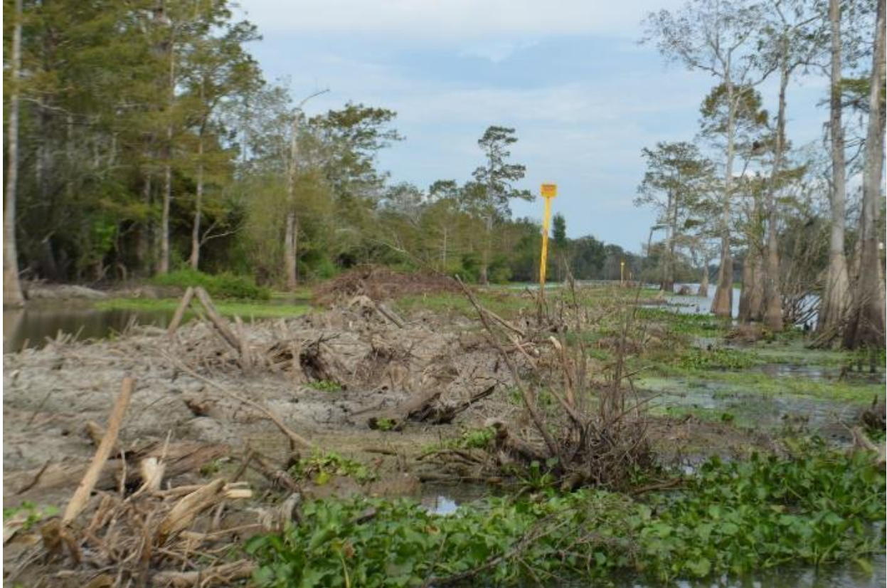
Fig. 4-E. This photo depicts illegal fill/Clean Water Act violations, dredged material/dirt/spoil and debris remaining along the pipeline right-of-way after construction and pipeline markers placed inside new spoil created by BBP. Dirt seen in the adjoining the forest to the left side of the photo may likely have been the result digging/dredging during high water without using appropriate, required erosion controls. Dean took this photo facing east, at a location east of Cross Bayou between the following approximate coordinates: 30° 05'12.84" N, 91°22'38.47" W and 30° 05'10.71" N, 91° 23'51.29" W.
